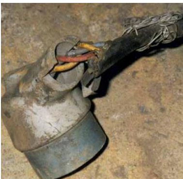
Damaged cable grip
